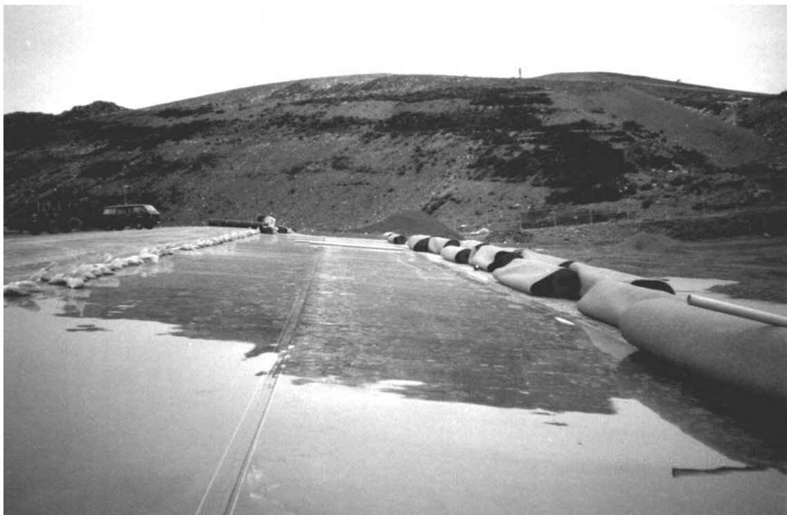
Figure 6. Example of a flat geomembrane on a landfill bottom.
